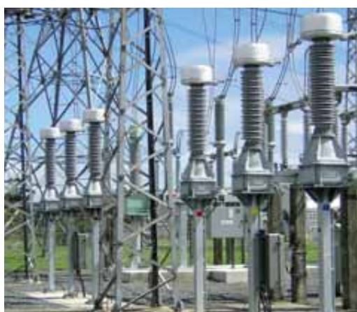
2. 123 kV Inductive voltage transformers. Transpower (New Zealand).
