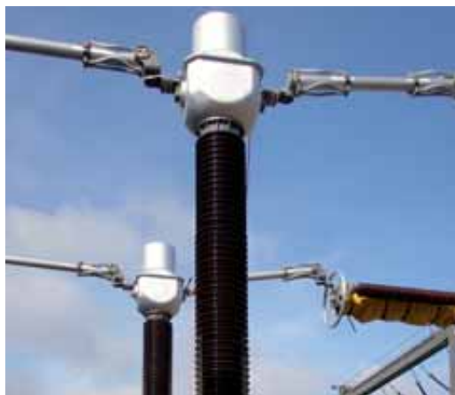
3. 420 kV Current transformers. National Grid (UK).
