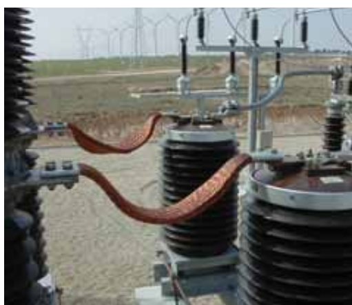
> 72.5 kV Current transformer (CX) used for wind farm substation protection. Iberdrola (Spain).
